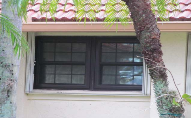
PROTECTED WITH UNVERIFIED SHUTTERS
