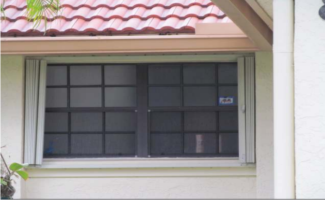
PROTECTED WITH UNVERIFIED SHUTTERS
