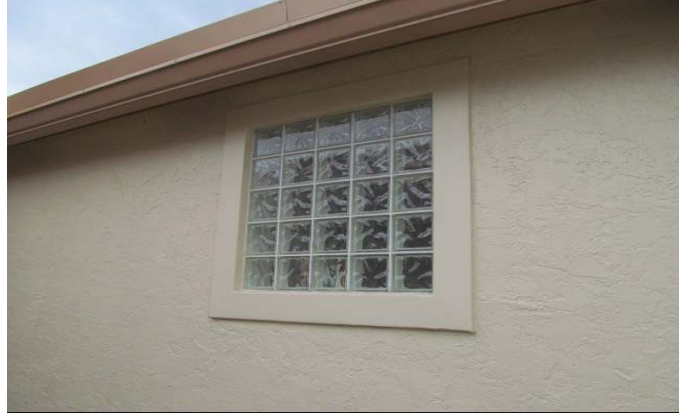
UNPROTECTED GLASS BLOCK
