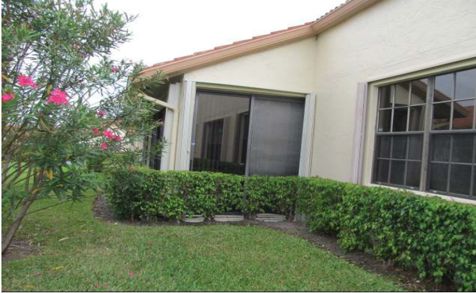
PROTECTED WITH UNVERIFIED SHUTTERS
