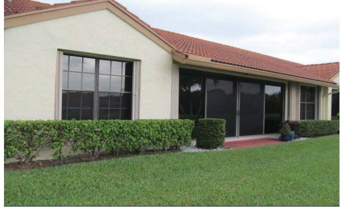
PROTECTED WITH UNVERIFIED SHUTTERS
