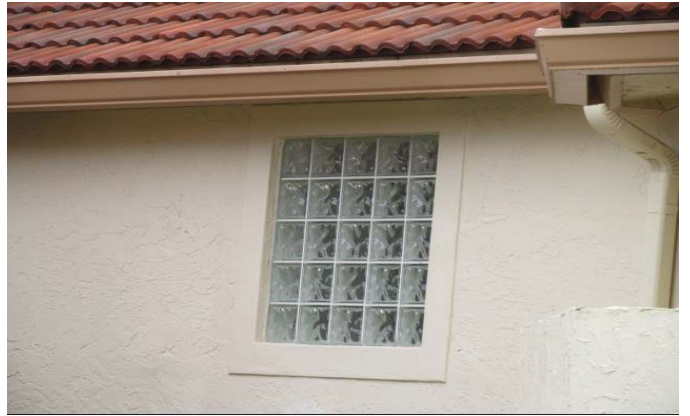
UNPROTECTED GLASS BLOCK
