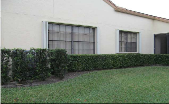
PROTECTED WITH UNVERIFIED SHUTTERS
