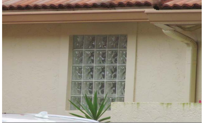
UNPROTECTED GLASS BLOCK
