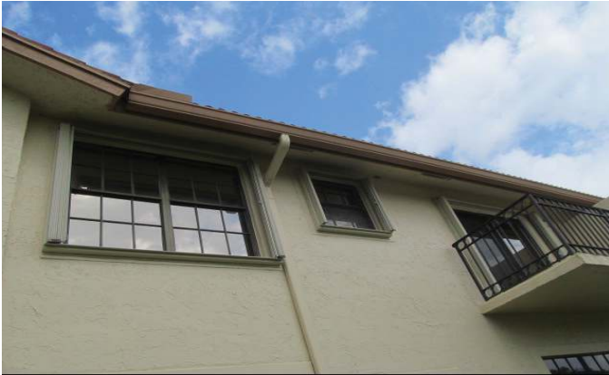
PROTECTED WITH UNVERIFIED SHUTTERS
