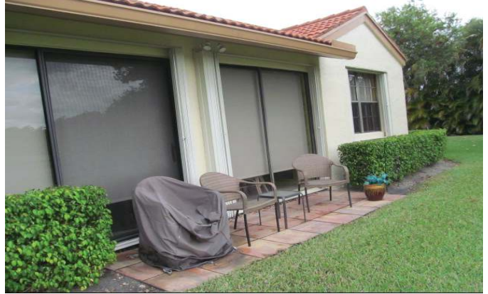
PROTECTED WITH UNVERIFIED SHUTTERS
