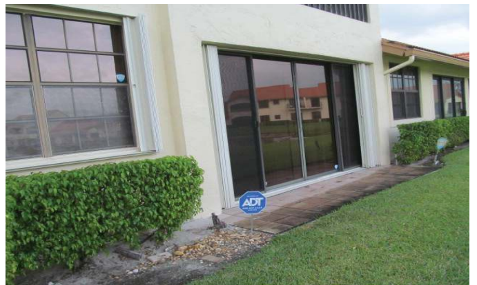
PROTECTED WITH UNVERIFIED SHUTTERS
