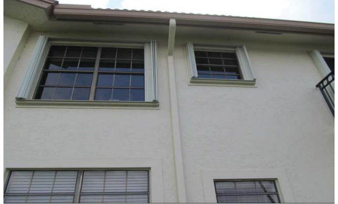
PROTECTED WITH UNVERIFIED SHUTTERS
