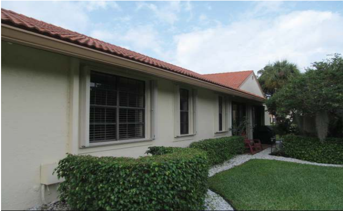
PROTECTED WITH UNVERIFIED SHUTTERS
