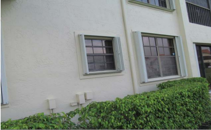
PROTECTED WITH UNVERIFIED SHUTTERS
