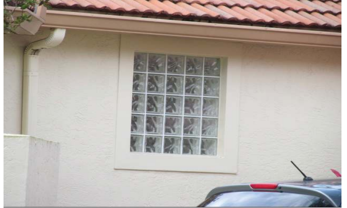
UNPROTECTED GLASS BLOCK
