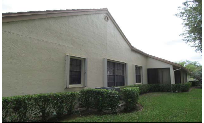
PROTECTED WITH UNVERIFIED SHUTTERS
