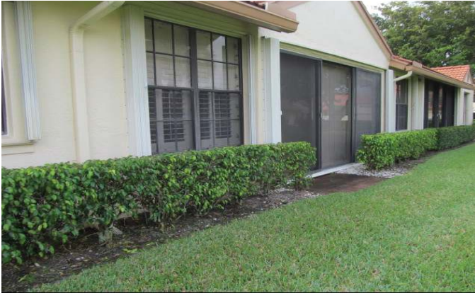
PROTECTED WITH UNVERIFIED SHUTTERS
