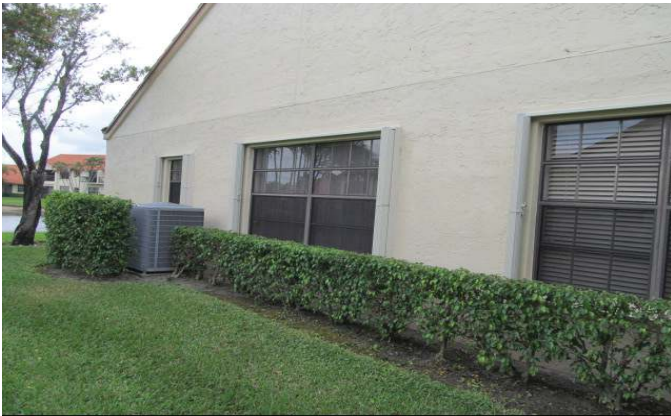
PROTECTED WITH UNVERIFIED SHUTTERS
