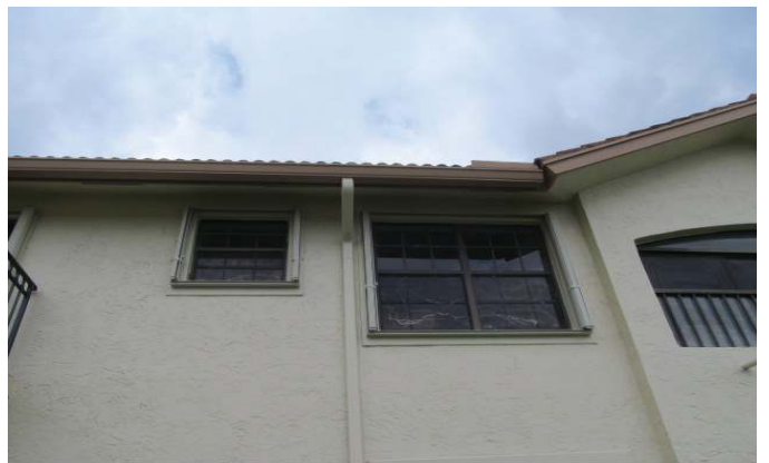
PROTECTED WITH UNVERIFIED SHUTTERS
