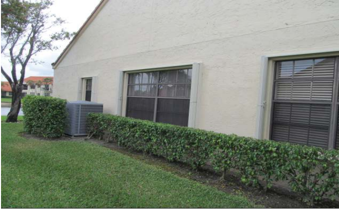
PROTECTED WITH UNVERIFIED SHUTTERS
