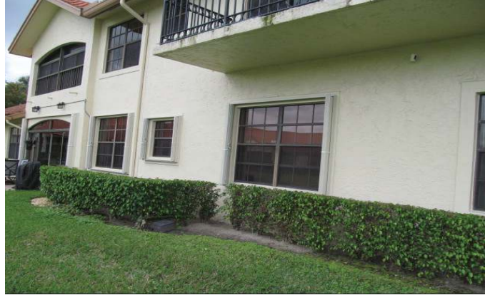
PROTECTED WITH UNVERIFIED SHUTTERS
