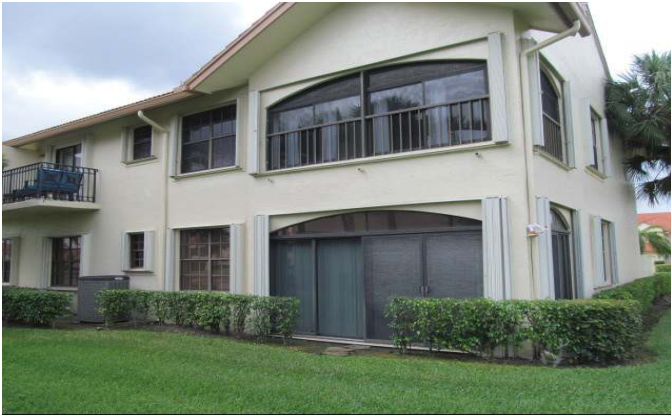
PROTECTED WITH UNVERIFIED SHUTTERS
