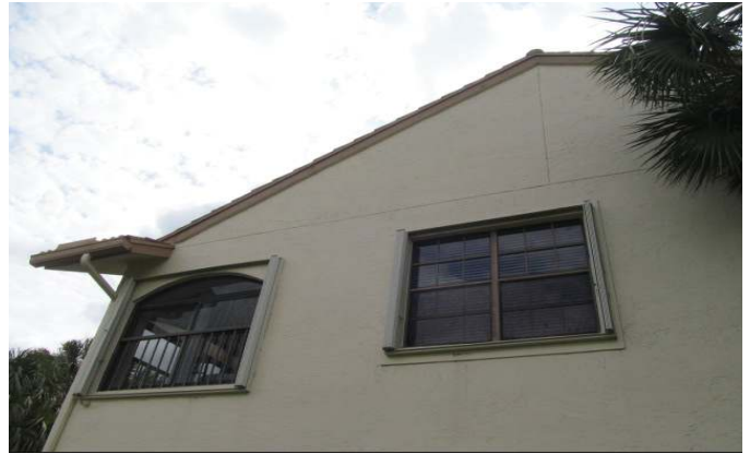
PROTECTED WITH UNVERIFIED SHUTTERS
