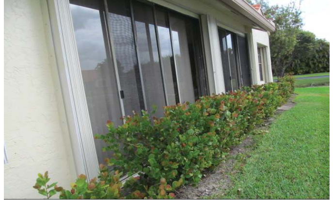
PROTECTED WITH UNVERIFIED SHUTTERS
