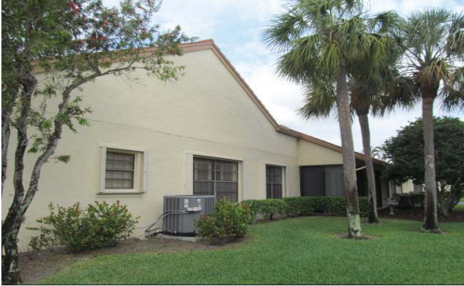
PROTECTED WITH UNVERIFIED SHUTTERS
