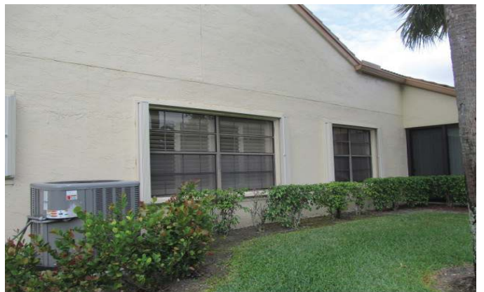
PROTECTED WITH UNVERIFIED SHUTTERS
