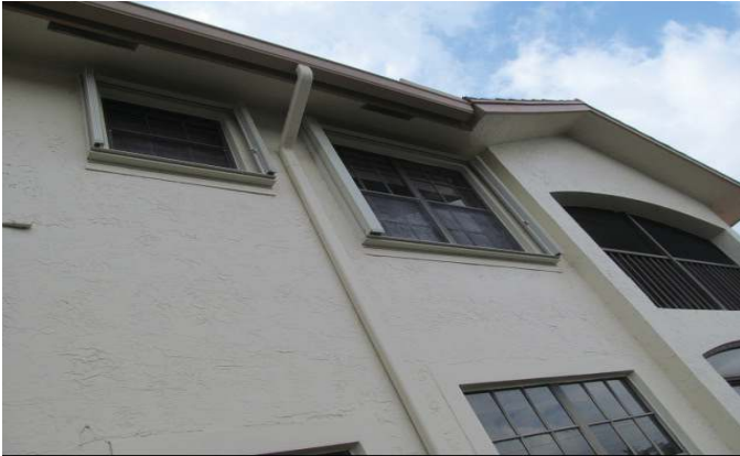
PROTECTED WITH UNVERIFIED SHUTTERS
