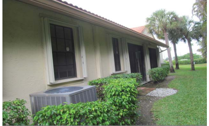
PROTECTED WITH UNVERIFIED SHUTTERS
