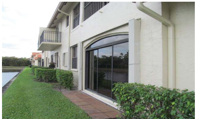
PROTECTED WITH UNVERIFIED SHUTTERS
