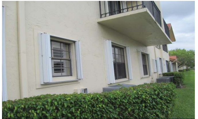
PROTECTED WITH UNVERIFIED SHUTTERS
