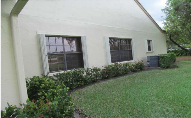
PROTECTED WITH UNVERIFIED SHUTTERS
