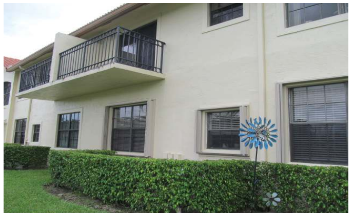
PROTECTED WITH UNVERIFIED SHUTTERS
