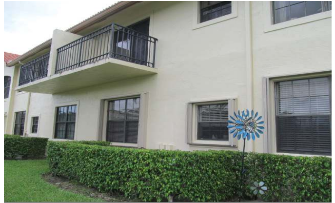
PROTECTED WITH UNVERIFIED SHUTTERS
