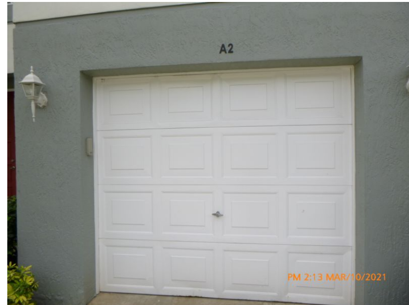
Unprotected Solid Garage Door
