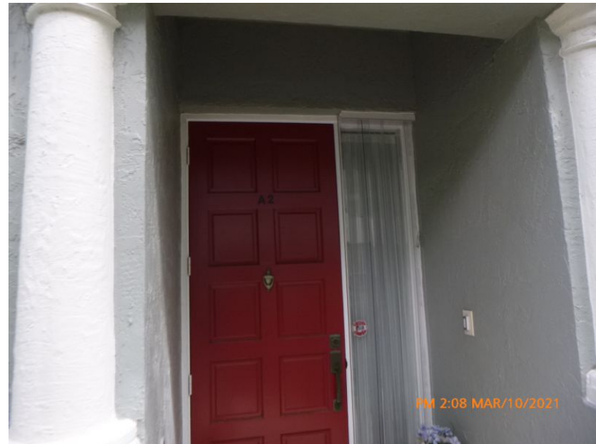
Unprotected Solid Entry Door
