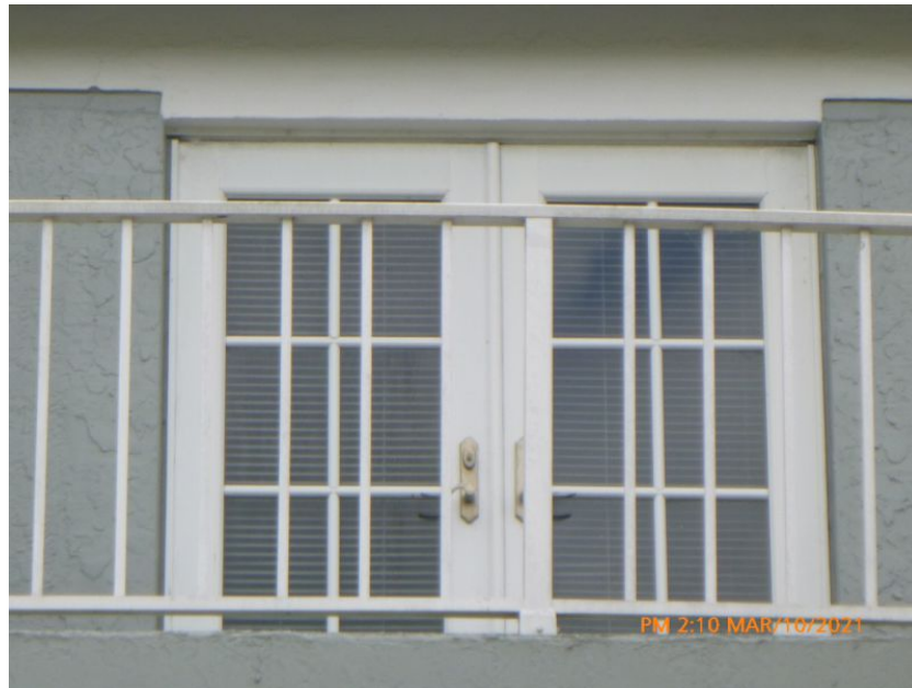
Unprotected Glazed Entry Door
