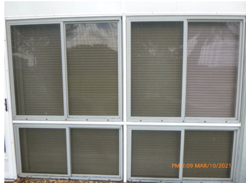
Unprotected Glazed Entry Door
