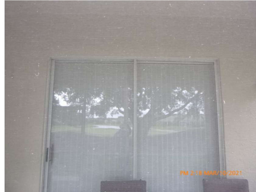
Unprotected Glazed Entry Door
