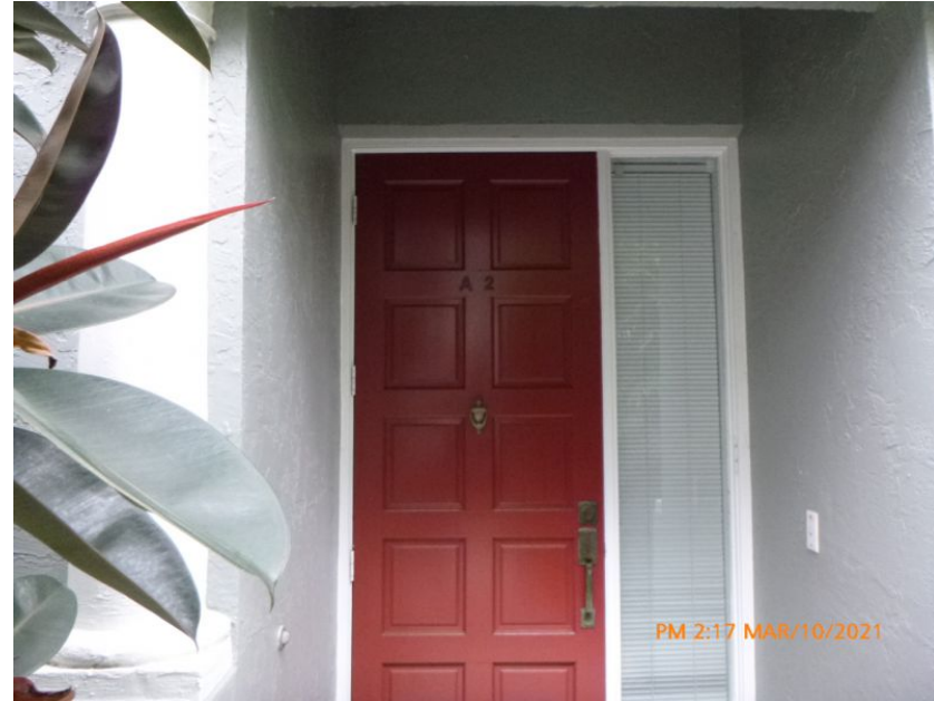
Unprotected Solid Entry Door
