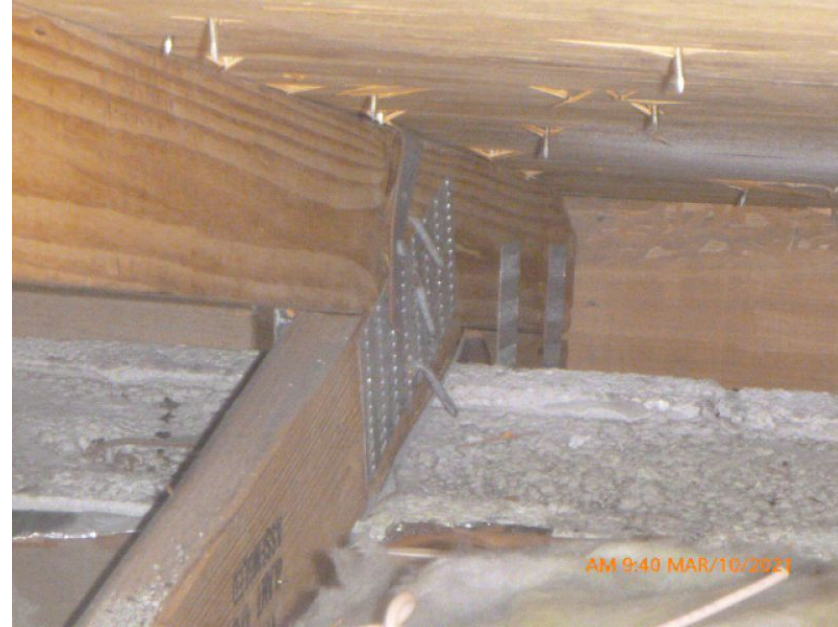
Metal Connector with Gap Greater than 1/2" from Truss
