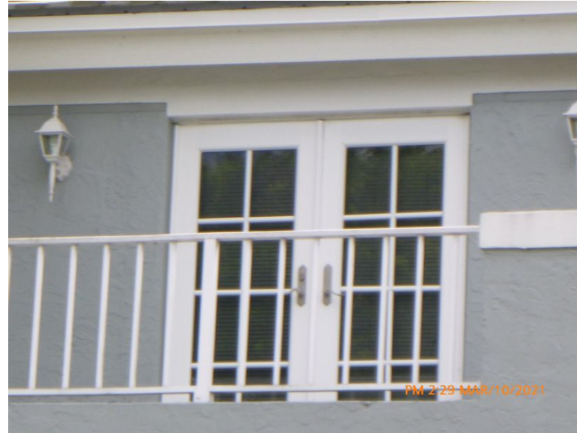
Unprotected Glazed Entry Door
