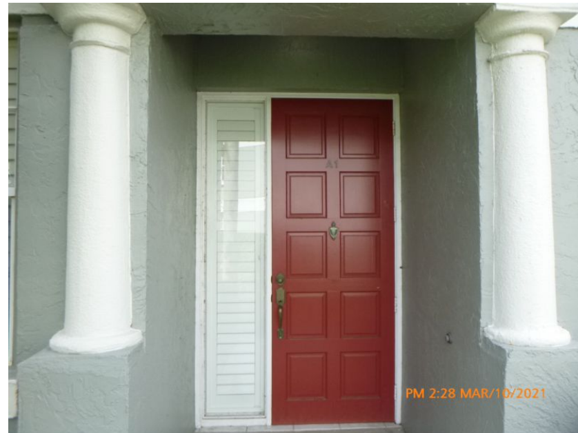
Unprotected Solid Entry Door
