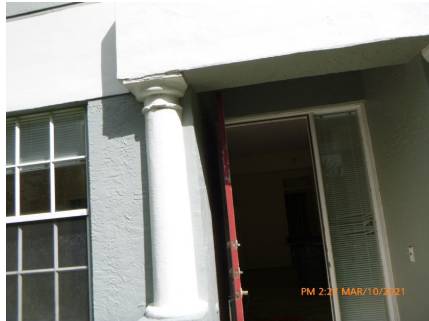
Unprotected Solid Entry Door
