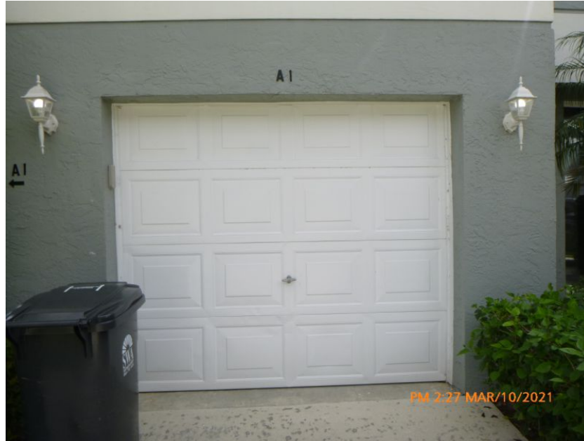
Unprotected Solid Garage Door
