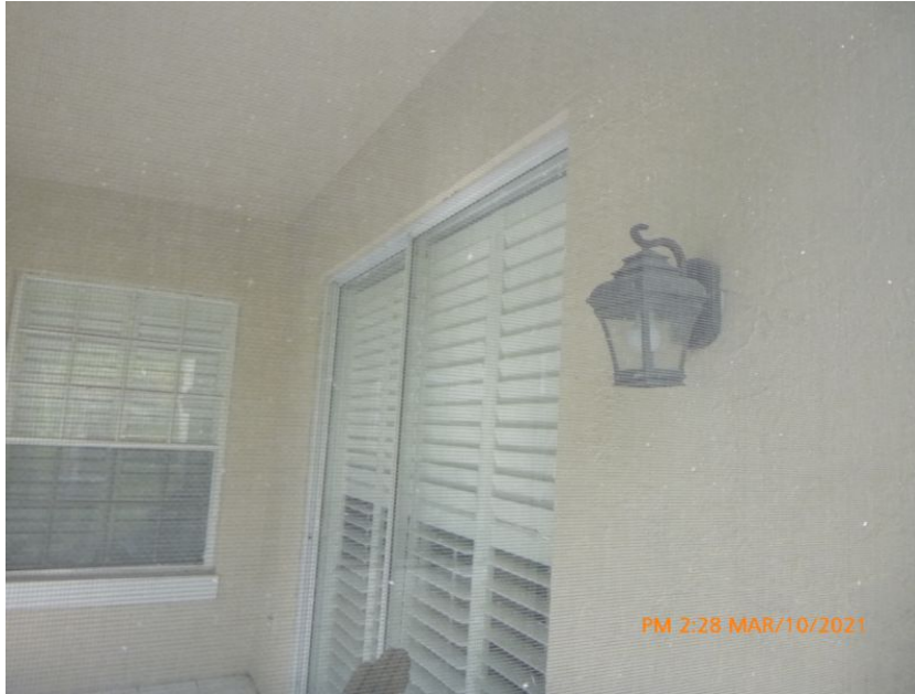
Unprotected Glazed Entry Door
