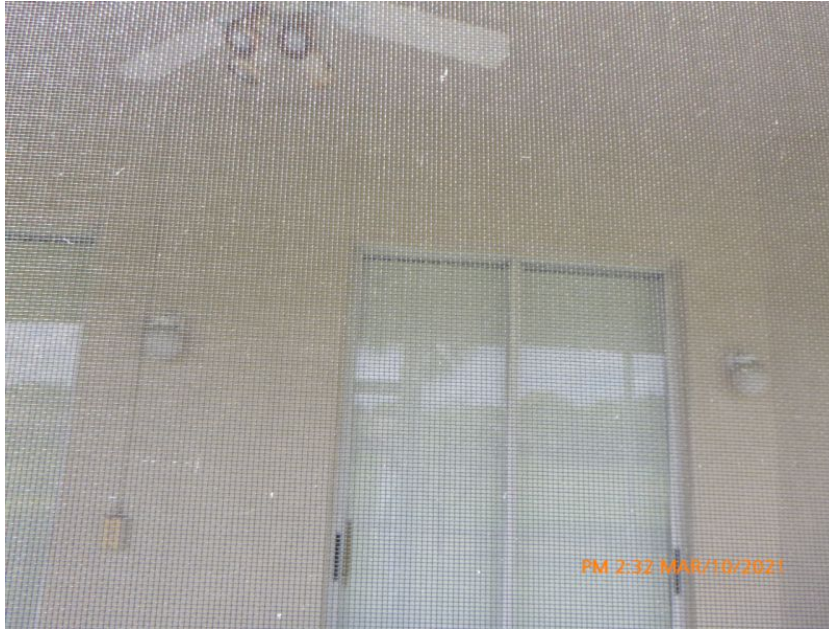
Unprotected Glazed Entry Door
