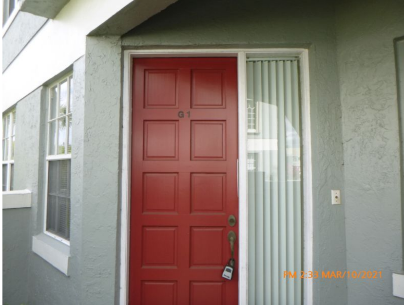
Unprotected Solid Entry Door
