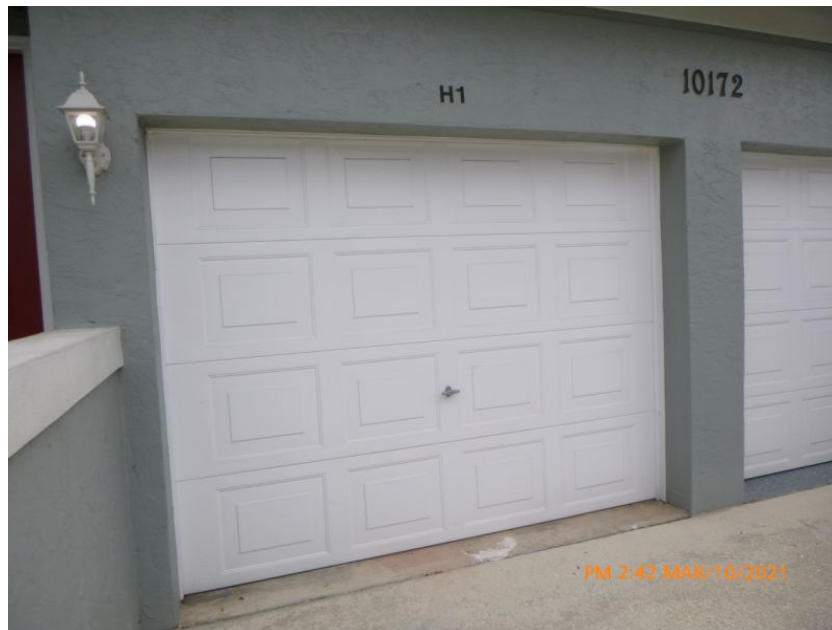
Unprotected Solid Garage Door
