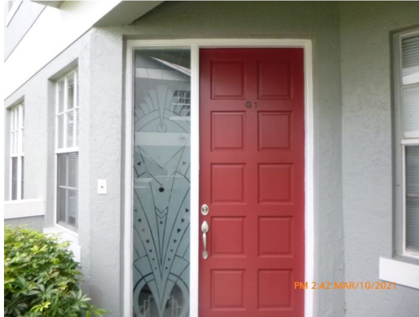
Unprotected Solid Entry Door
