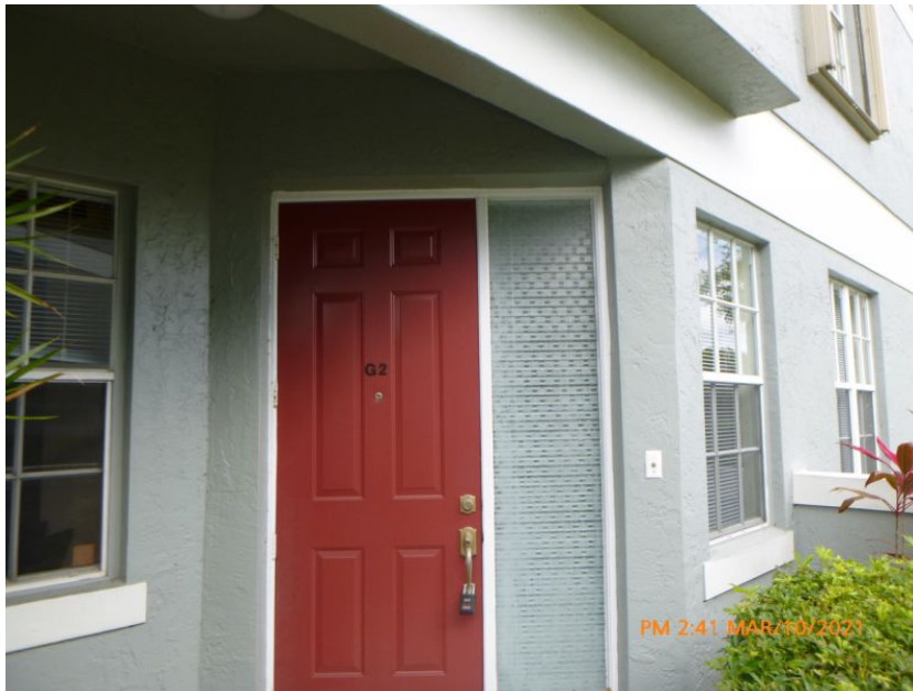
Unprotected Solid Entry Door
