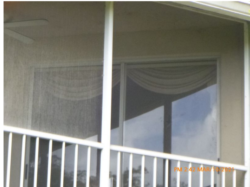
Unprotected Glazed Entry Door
