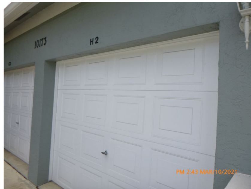
Unprotected Solid Garage Door
