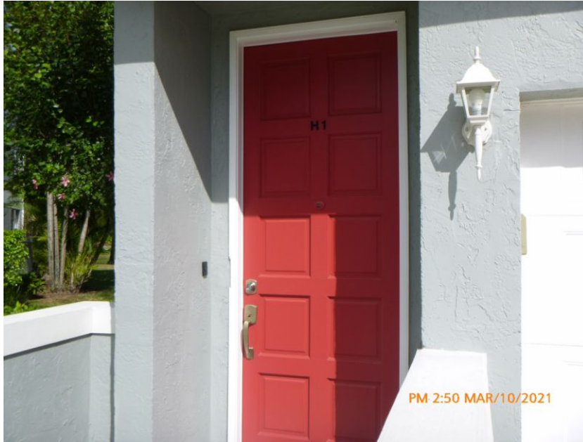
Unprotected Solid Entry Door
