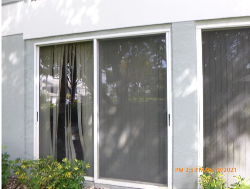
Unprotected Glazed Entry Door
