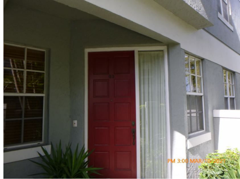
Unprotected Solid Entry Door
