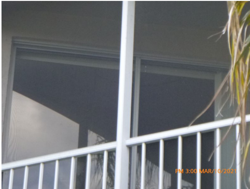
Unprotected Glazed Entry Door
