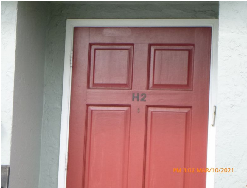
Unprotected Solid Entry Door
