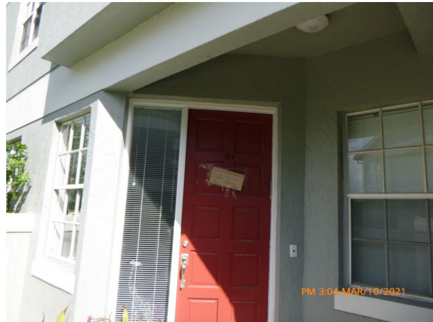
Unprotected Solid Entry Door
