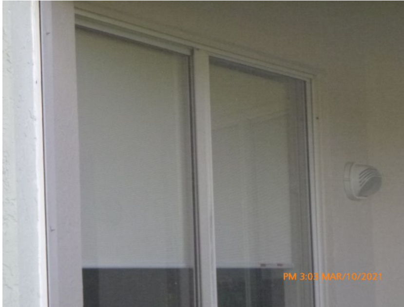
Unprotected Glazed Entry Door
