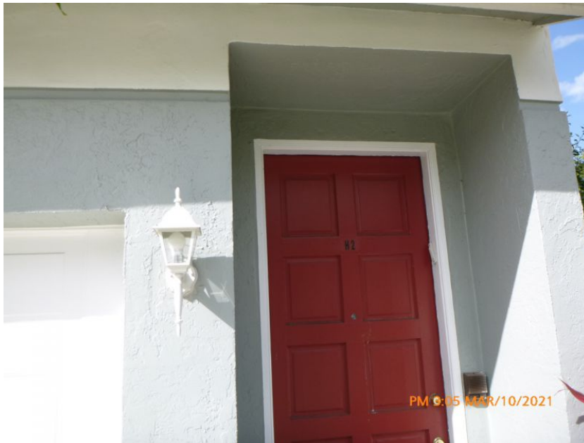
Unprotected Solid Entry Door
