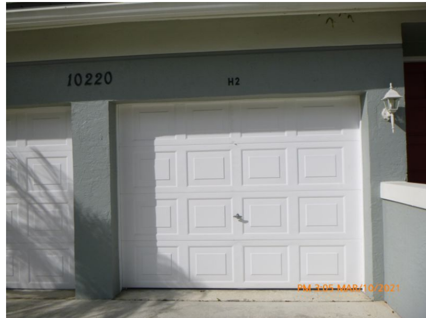
Unprotected Solid Garage Door
