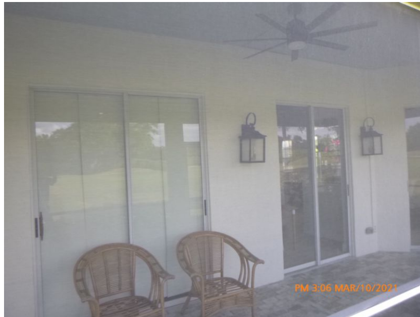
Unprotected Glazed Entry Door
