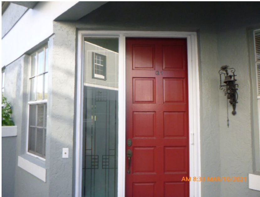
Unprotected Solid Entry Door
