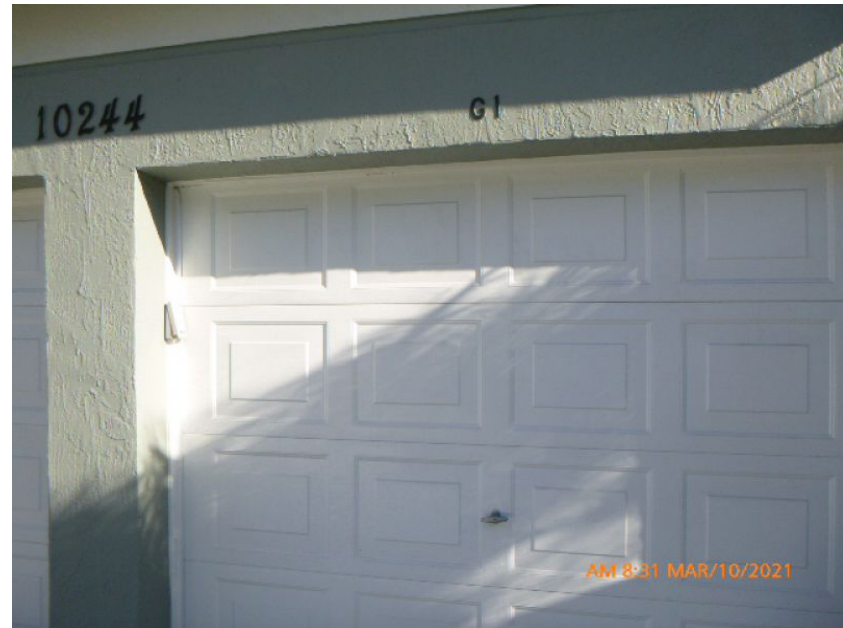
Unprotected Solid Garage Door
