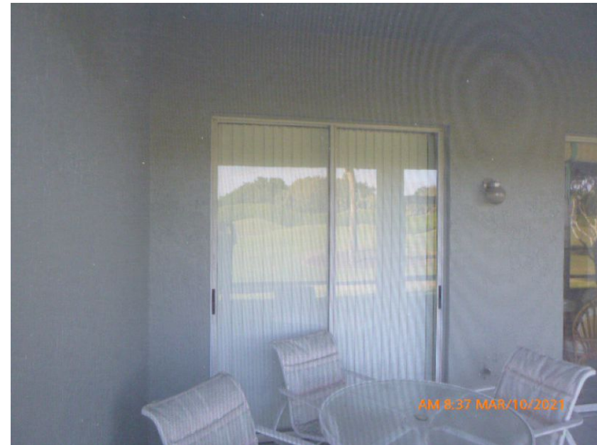
Unprotected Glazed Entry Door
