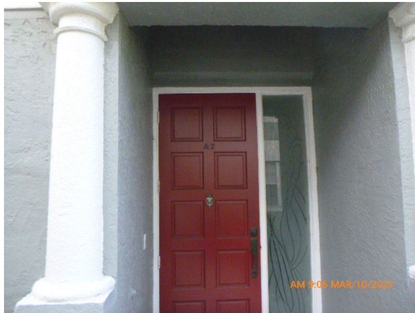
Unprotected Solid Entry Door
