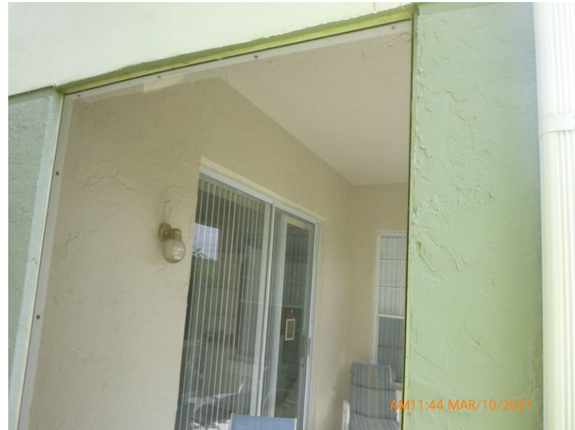
Unprotected Glazed Entry Door
