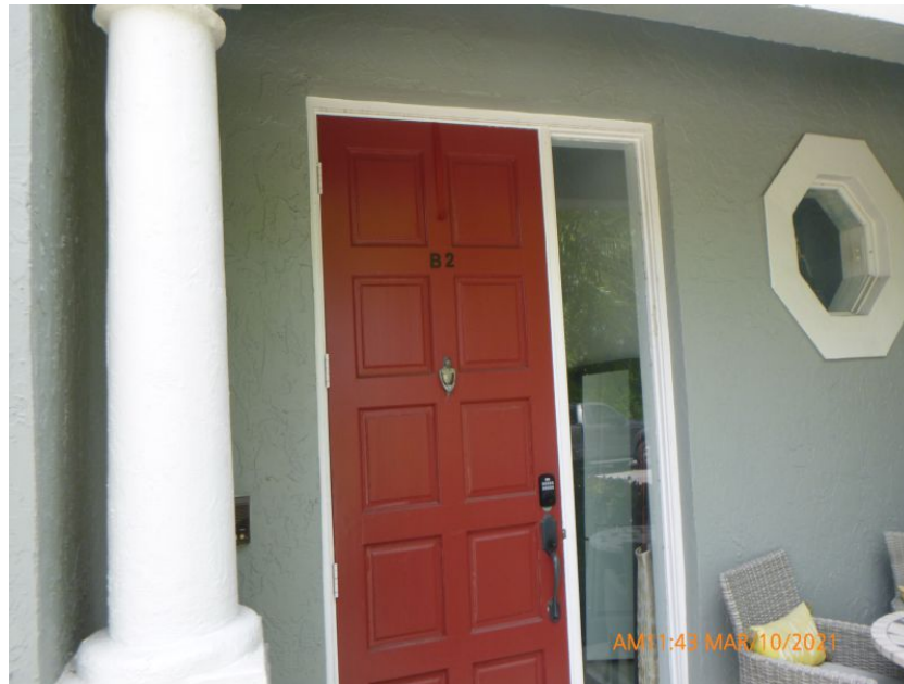
Unprotected Solid Entry Door
