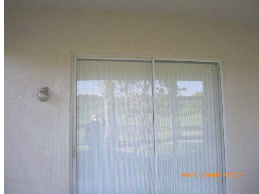
Unprotected Glazed Entry Door
