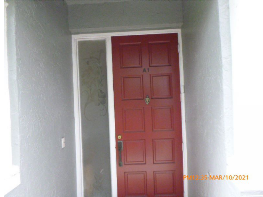
Unprotected Solid Entry Door
