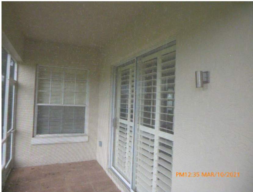
Unprotected Glazed Entry Door
