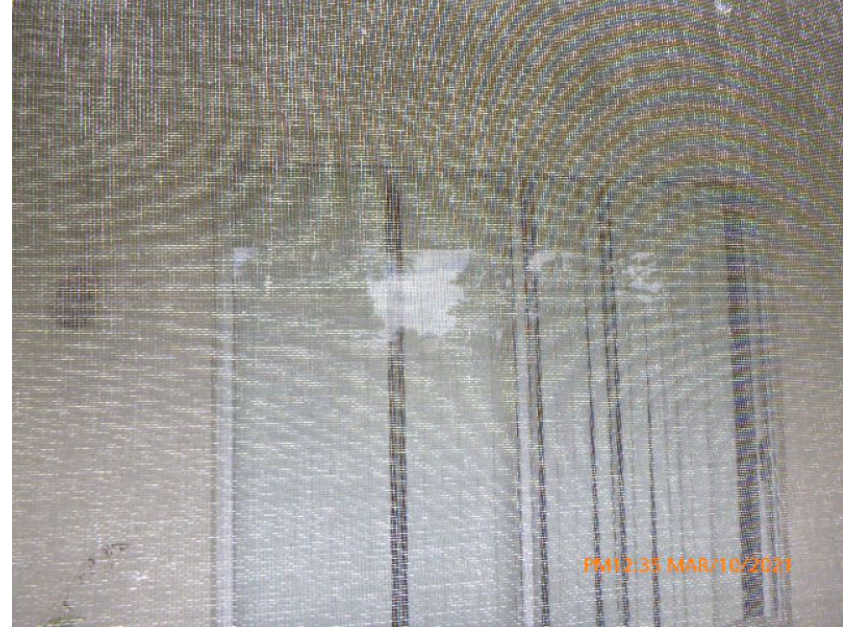
Unprotected Glazed Entry Door
