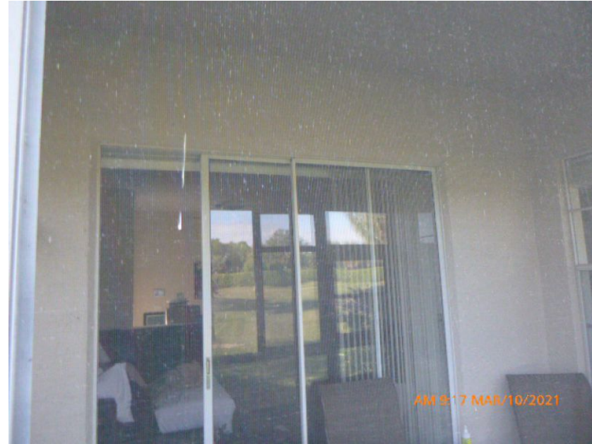
Unprotected Glazed Entry Door
