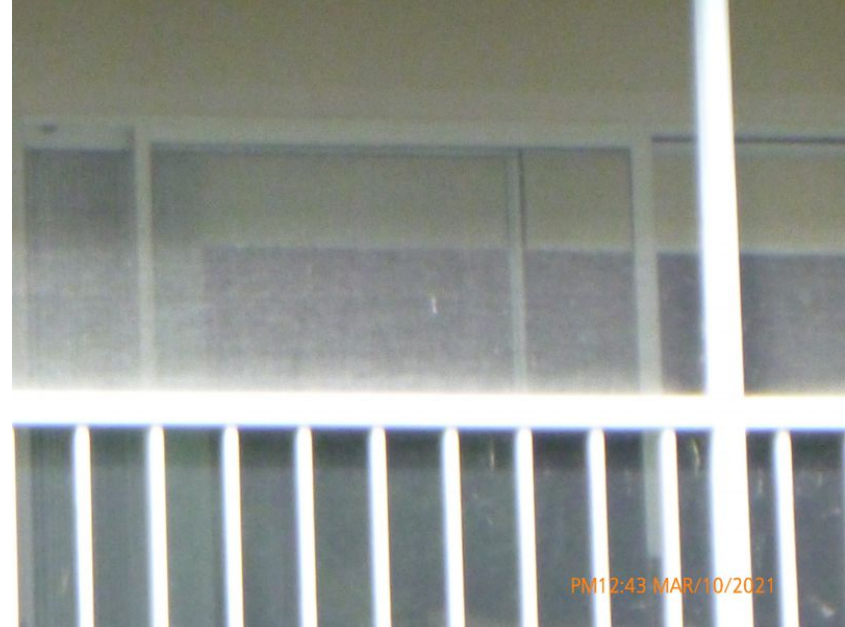
Unprotected Glazed Entry Door
