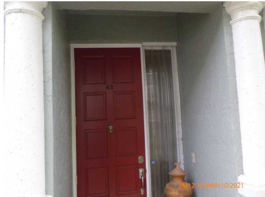
Unprotected Solid Entry Door
