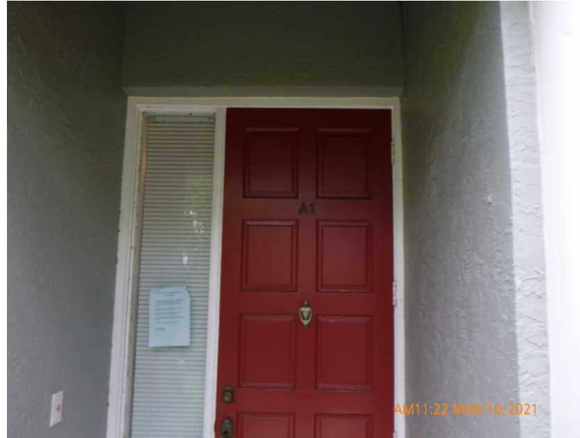
Unprotected Solid Entry Door
