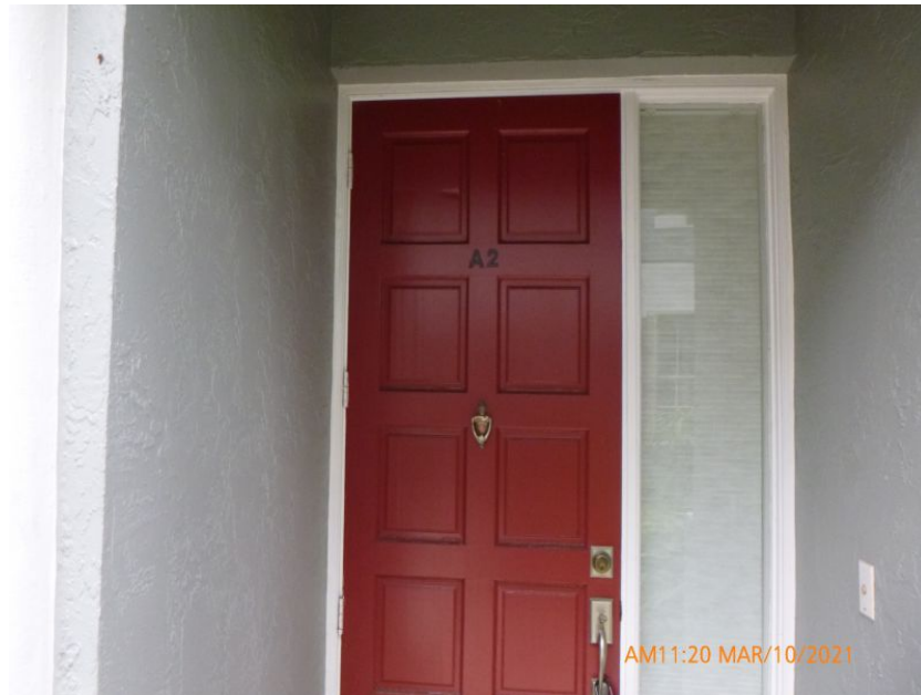
Unprotected Solid Entry Door
