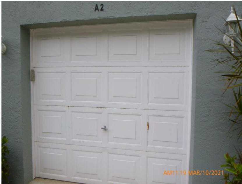
Unprotected Solid Garage Door
