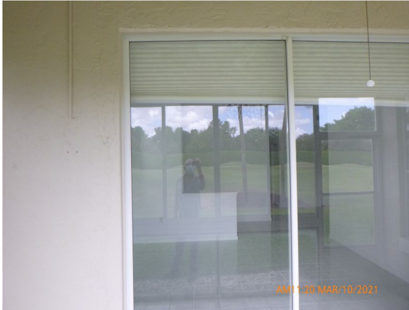
Unprotected Glazed Entry Door
