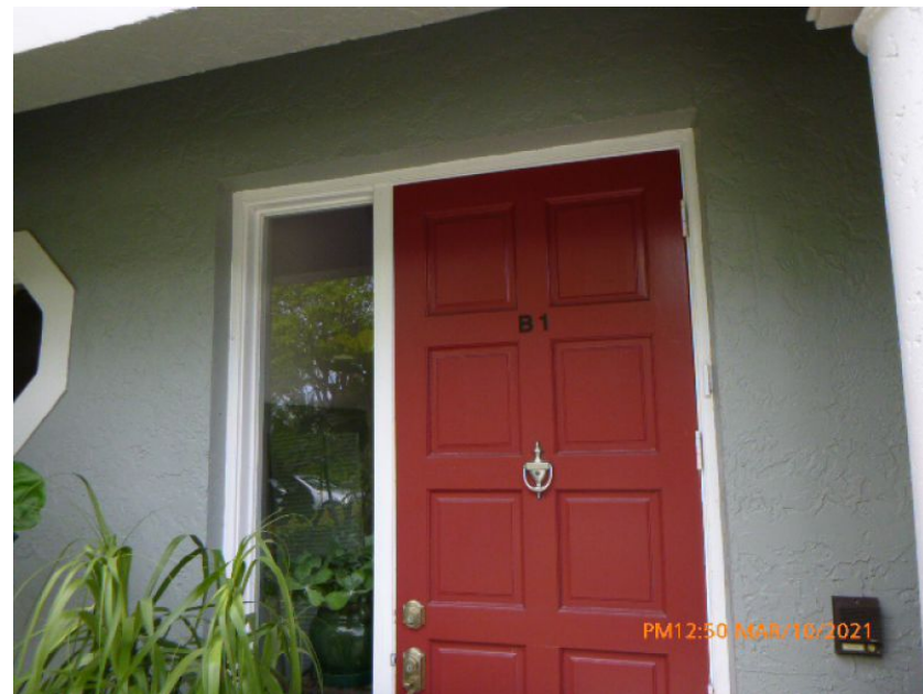
Unprotected Solid Entry Door
