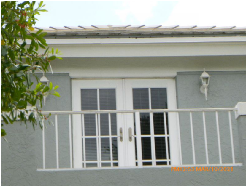
Unprotected Glazed Entry Door
