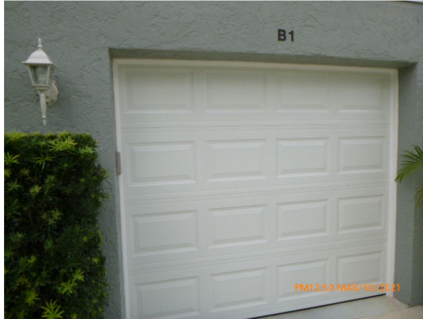
Unprotected Solid Garage Door
