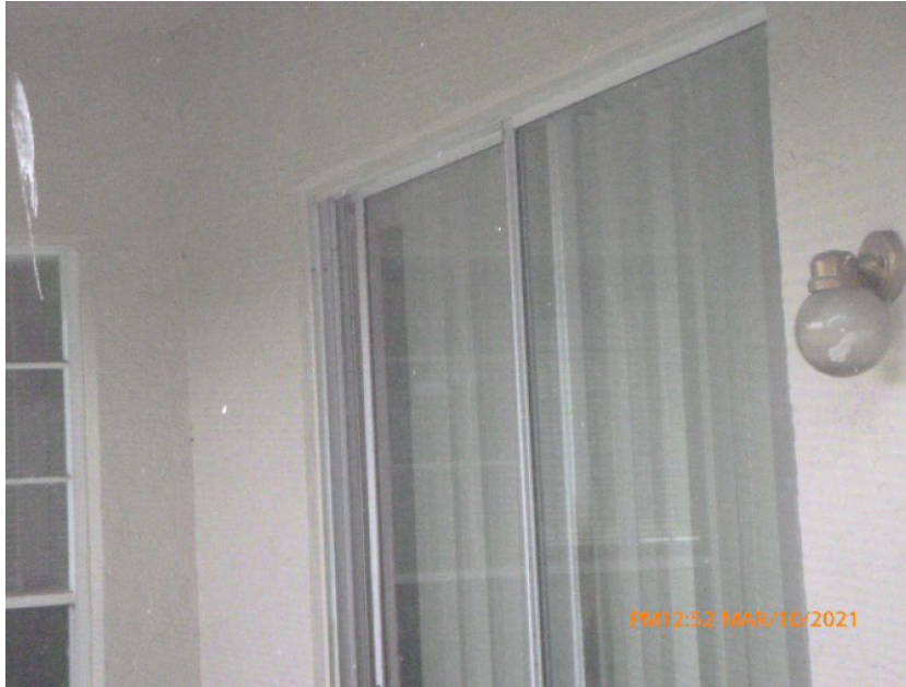
Unprotected Glazed Entry Door
