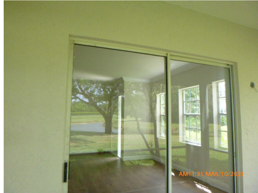
Unprotected Glazed Entry Door
