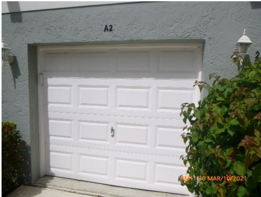
Unprotected Solid Garage Door
