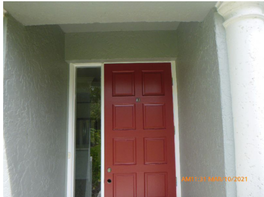
Unprotected Solid Entry Door
